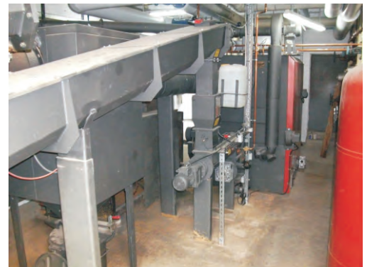
Fuel feeding and separate de-duster (heat insulated) incl. induced draught and a dust bin that is easily to change
